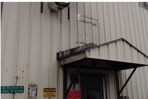
PATCHING AND CORROSION AT SIDING
