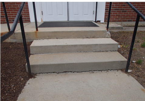
CRACK IN CONCRETE STAIR CORROSION AT DOOR FRAME
