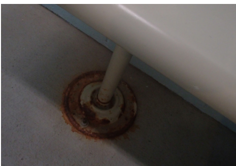
TYPICAL CORROSION AT BENCHES
