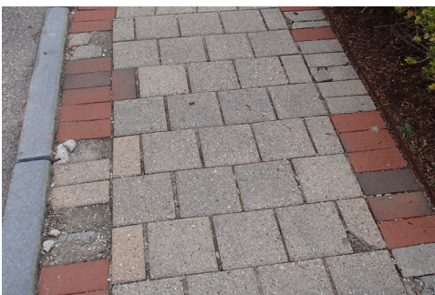
DAMAGED PAVERS WITH BRICK REPLACEMENTS
