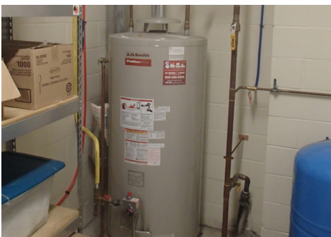
PLUMBING HOT WATER HEATER
