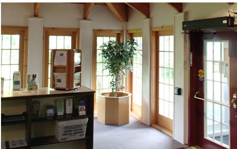
INTERIOR LOBBY FINISHES WORN & WORN FLOORING UNDER WALK OFF MAT
