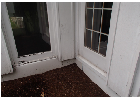
WATER DAMAGE AT WATER TABLE
