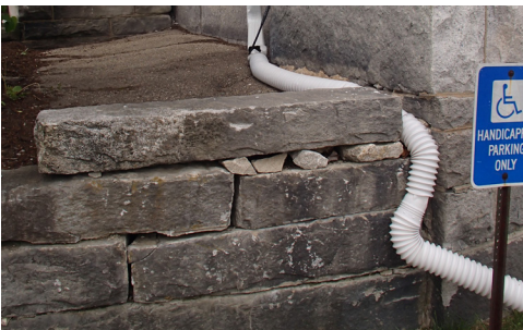
REPOINTING REQUIRED AT GRANITE
