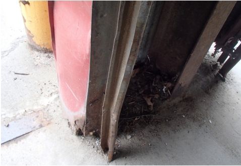
CORROSION AT DOOR FRAMES
