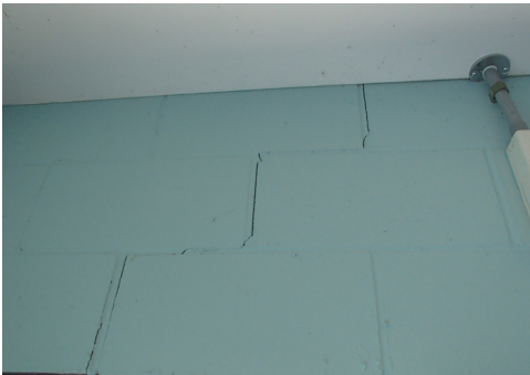
INTERNAL CMU CRACK AT DOOR HEAD
