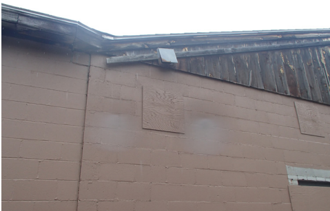
WEATHERED TRIM AT WINDOW BOARDING
