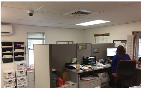
TYPICAL EXISTING LIGHTING, SURVEILLANCE CAMERA, & HVAC
