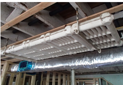
OLD AND NEW MECHANICAL SYSTEMS
