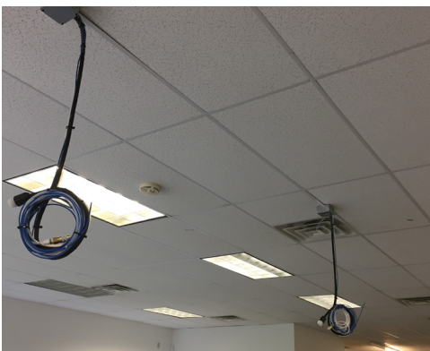
CORDS HANGING FROM CEILING
