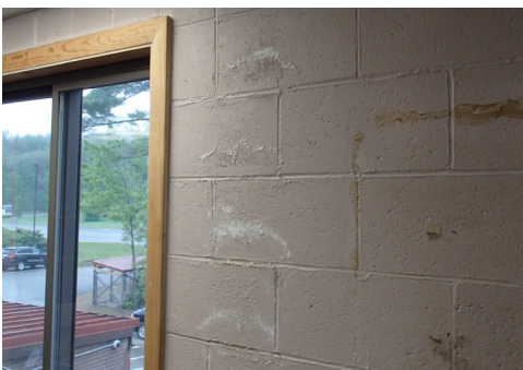
EFFLORESCENCE AT PERIMETER WALLS
