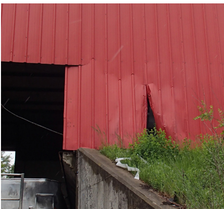
EXTERIOR SIDING DAMAGE
