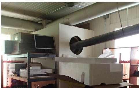
BOILER IN CLOSET WITH EXPOSED EXHAUST VENT
