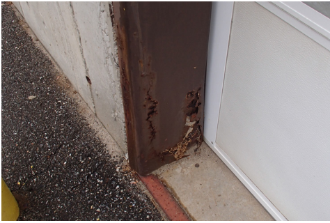
CORROSION AT DOOR FRAMES
