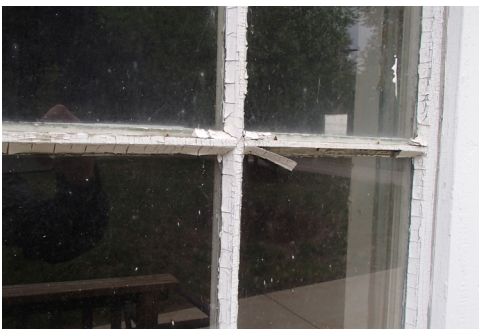
WINDOWS NEED REGLAZING
