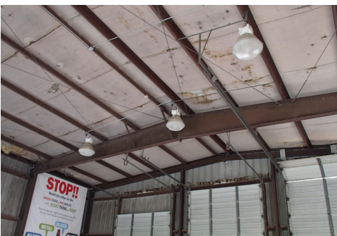
DAMAGED INSULATION AT CEILING
