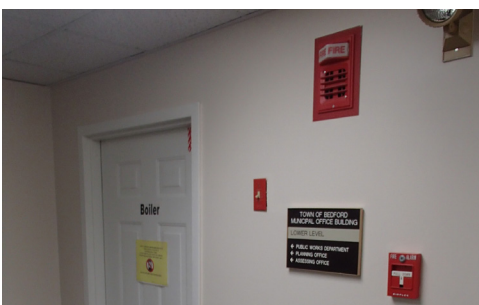
HORN STROBE, PULL STATION, AND OLDER EMERGENCY LIGHTING
