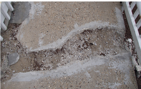
DAMAGE AT ADA ENTRY RAMP
