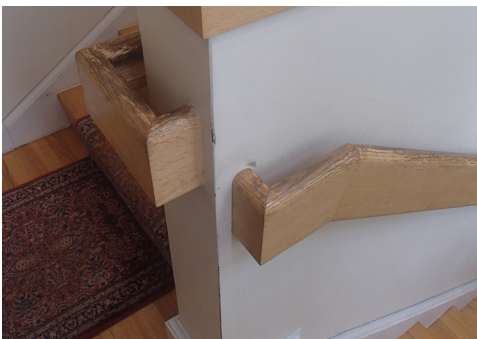
RAILING WEAR NON CONTINUOUS
