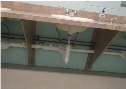
INSUFFICIENT ADA WRAP AT SINKS
