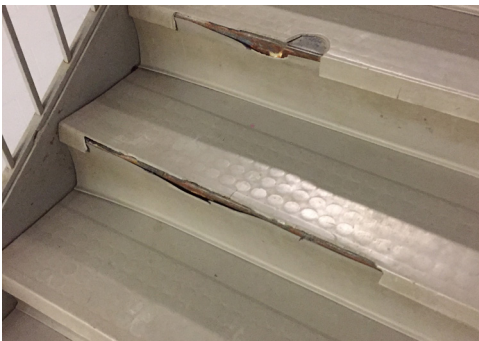
DAMAGED STAIR TREADS
