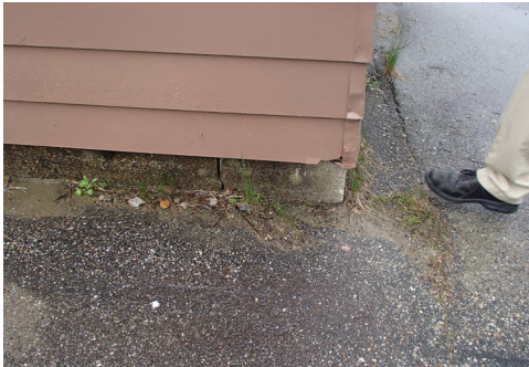
CORNER CRACK AT FOUNDATION
