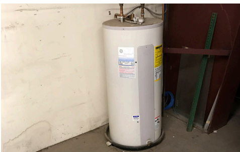
DOMESTIC HOT WATER HEATER
