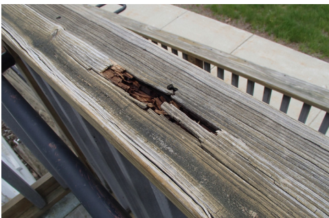
ROT AT WOOD HANDRAIL AT RAMP
