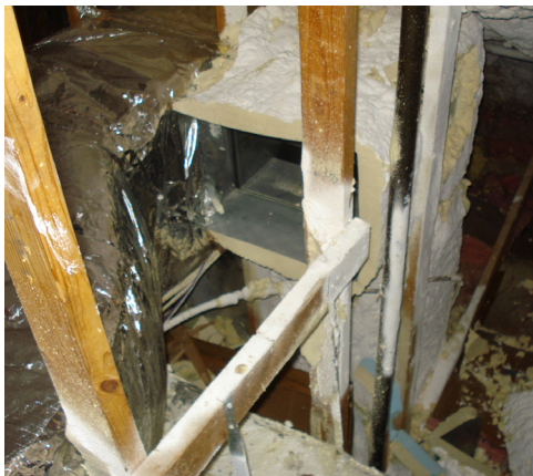
FOAM OVERSPRAY IN ATTIC
