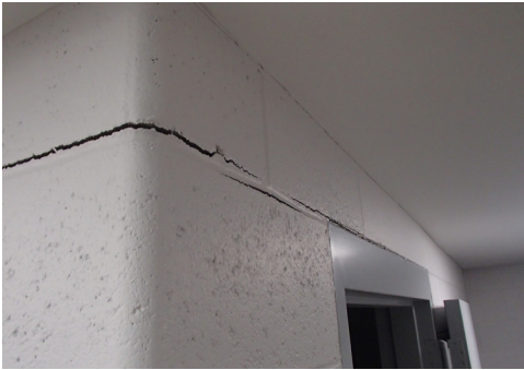
CRACKS IN CMU WALL
