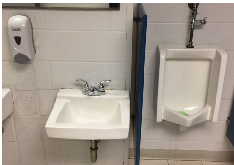
TYPICAL RESTROOM PLUMBING FIXTURES
