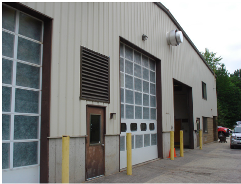
GRILLS/VENT FOR NEW CO SYSTEM
