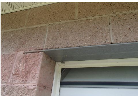
MORTAR CRACKS AT CMU
