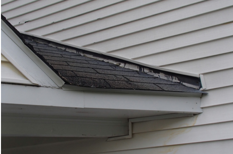
WORN ROOFING & FLASHING
