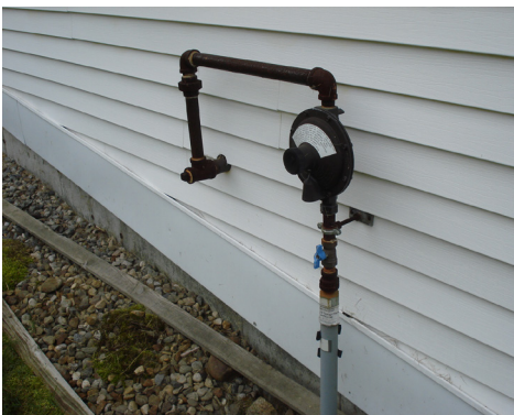
GAS SERVICE ENTRANCE
