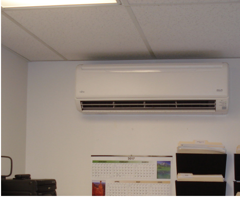
TYPICAL SPLIT SYSTEM IN OFFICE
