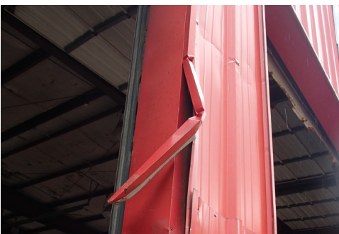
VEHICLE DAMAGE AT DOOR GARAGE OPENING
