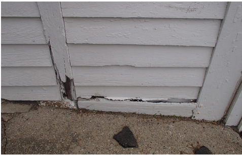
DAMAGE AT WOOD SIDING AND TRIM
