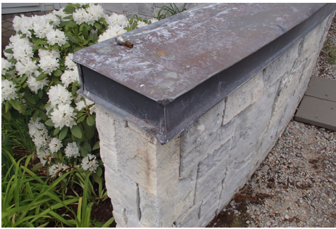
DAMAGE AT METAL FLASHING AND CAPS
