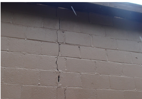
CRACK AT CMU WALL
