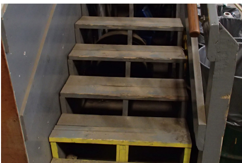
OPEN STAIR TREADS MISSING RAILING
