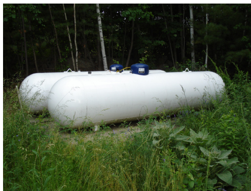
HEATING FUEL PROPANE TANKS
