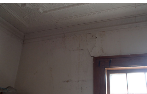
WATER DAMAGE AT INTERIOR WALLS
