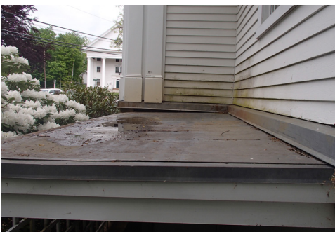
WATER DAMAGE AT SIDING POOLING IN ROOF
