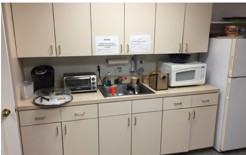
BREAK ROOM PLUMBING
