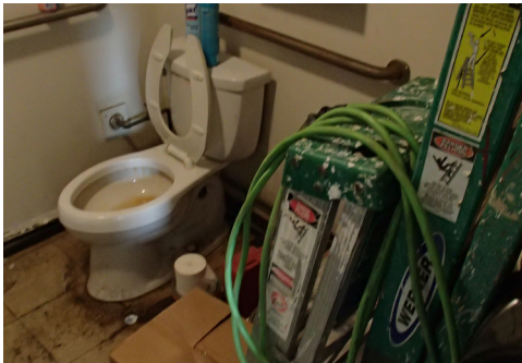
TYPICAL RESTROOM PLUMBING FIXTURES
