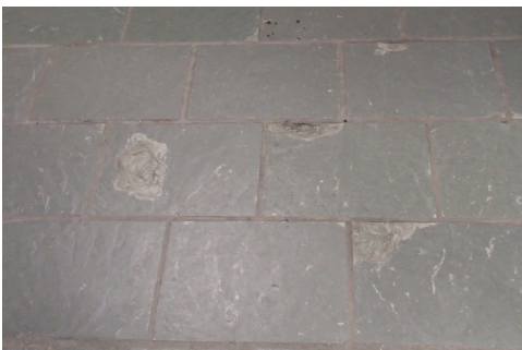
DAMAGE AT STONE FLOORING
