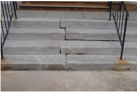
CORROSION AT ENTRANCE CONCRETE STAIR AND WOOD RAMP
