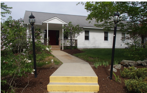
BUILDING EXTERIOR - NON-COMPLIANT BUILDING ACCESS
